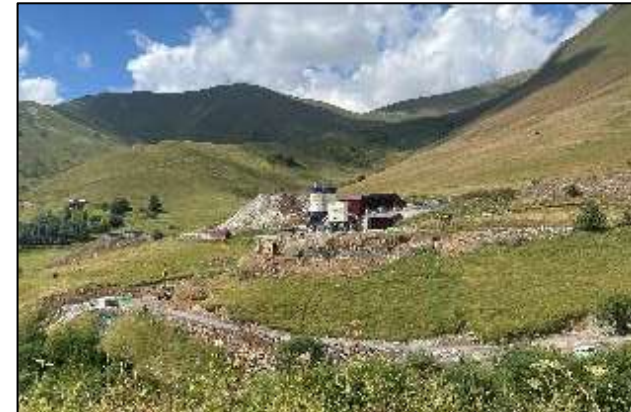
Lot 1: Tskere Batching Plant
